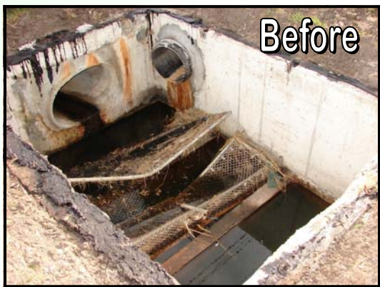
Broken screens made from chain link fence lay flat in the structure.
